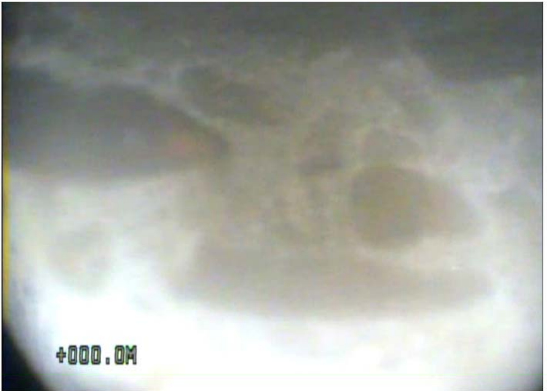
Concrete Rubble – Below Water
