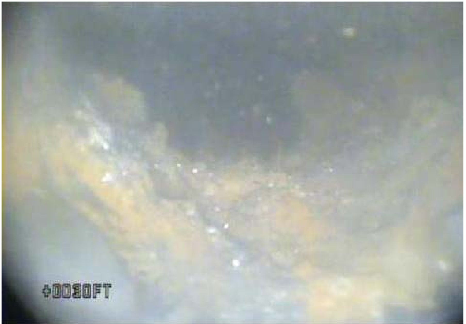
Weathered Bedrock and Large Void
