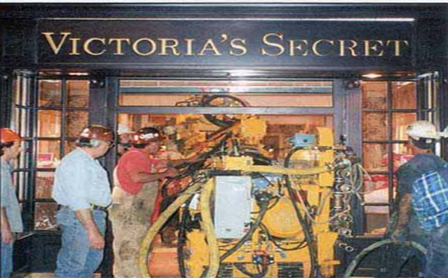
This night crew is not Christmas shopping; they are using pin piles to overcome difficult ground conditions and tight access requirements at an expansion of Exton Square Mall, in Exton, Pa. The construction team moves in specialized equipment to install piles at night; by morning, business in the store carried on as usual, without any evidence of drilling.
