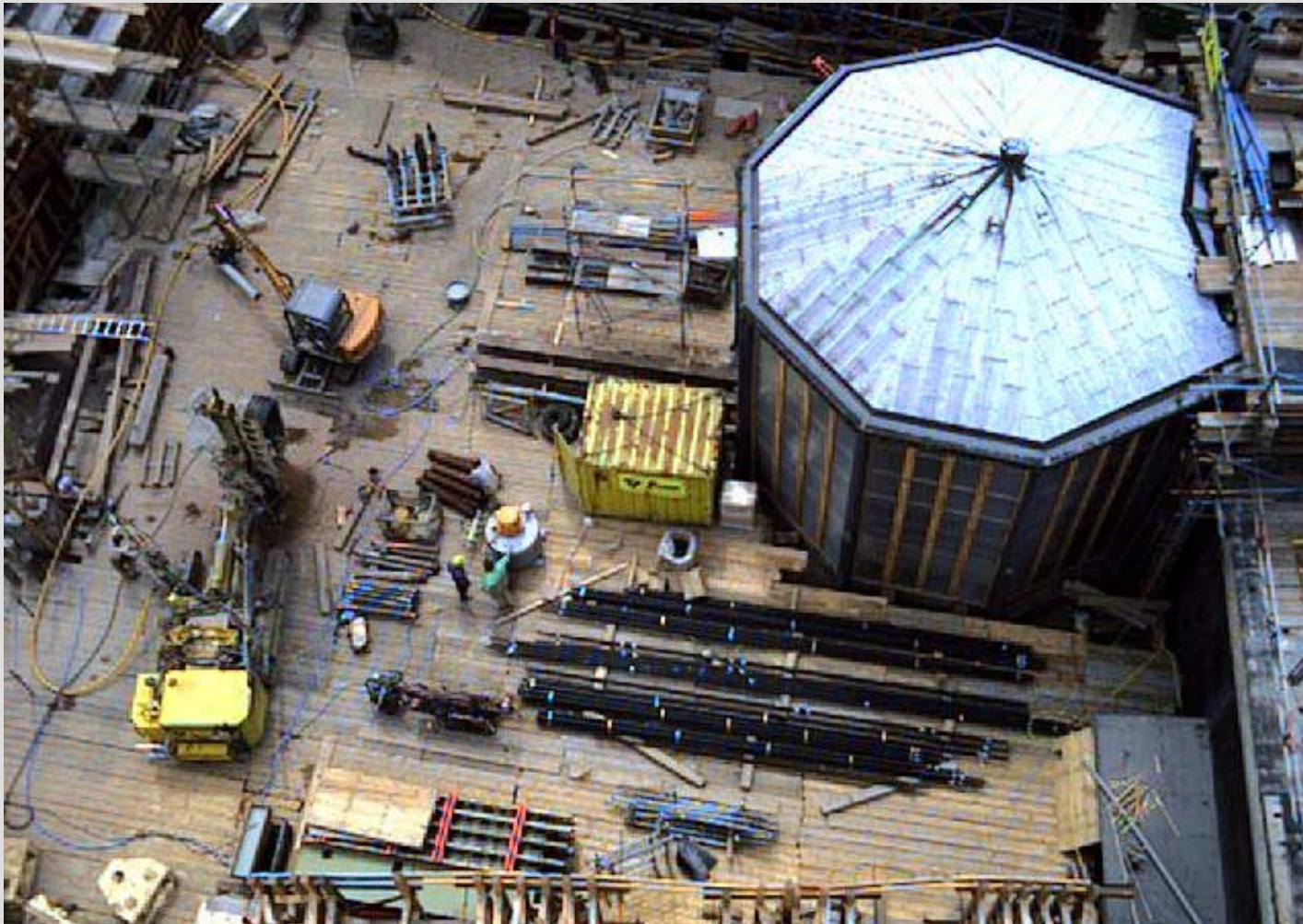
Drilling for micro piles at the chapel and on the digging field
