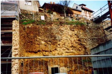
(photograph of deteriorated / decayed wall)
