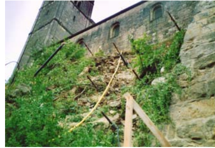
Anchors in slope
