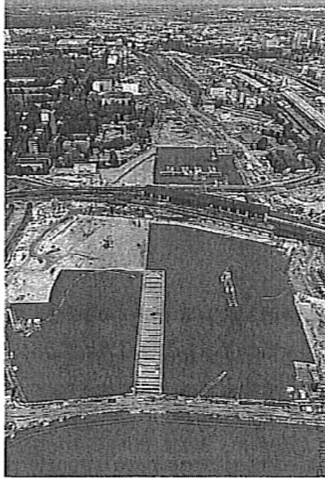
Fig. 5 Free ground water level with floating equipment for dredging and micropile installation (rear) at central site (Lehrter Bahnhof)
