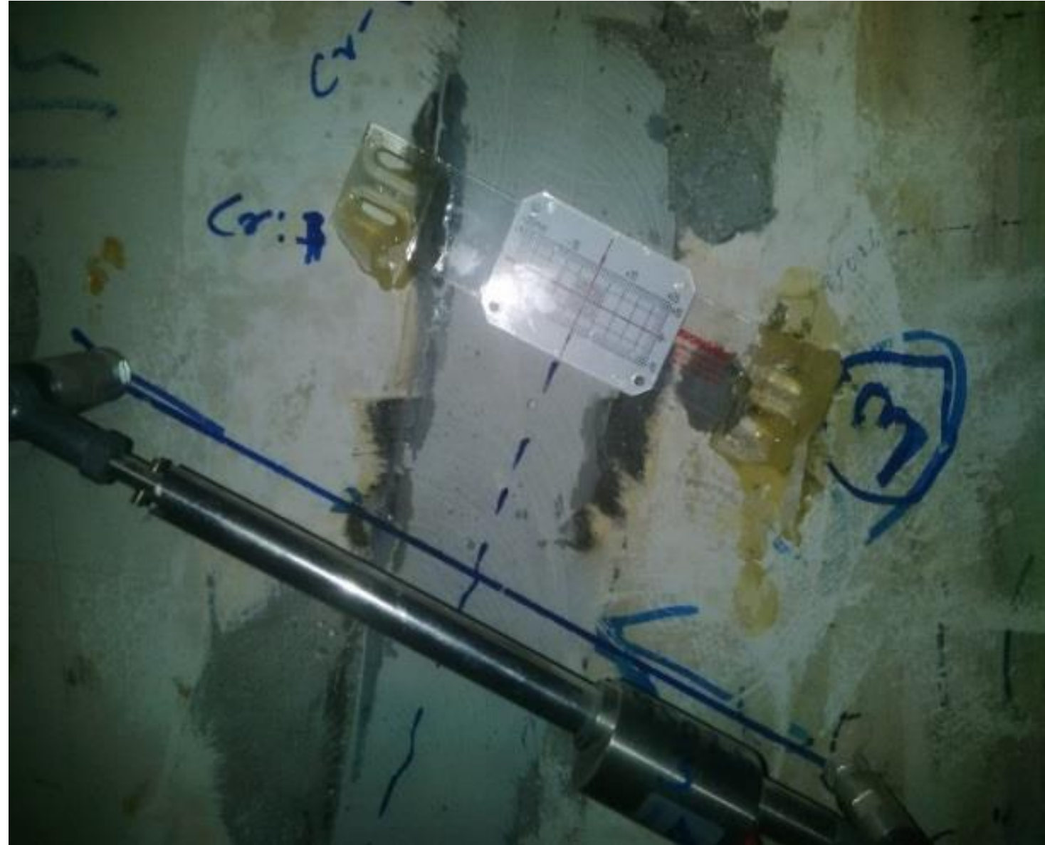
Figure 9: monitoring of cracks installed monitoring equipment
