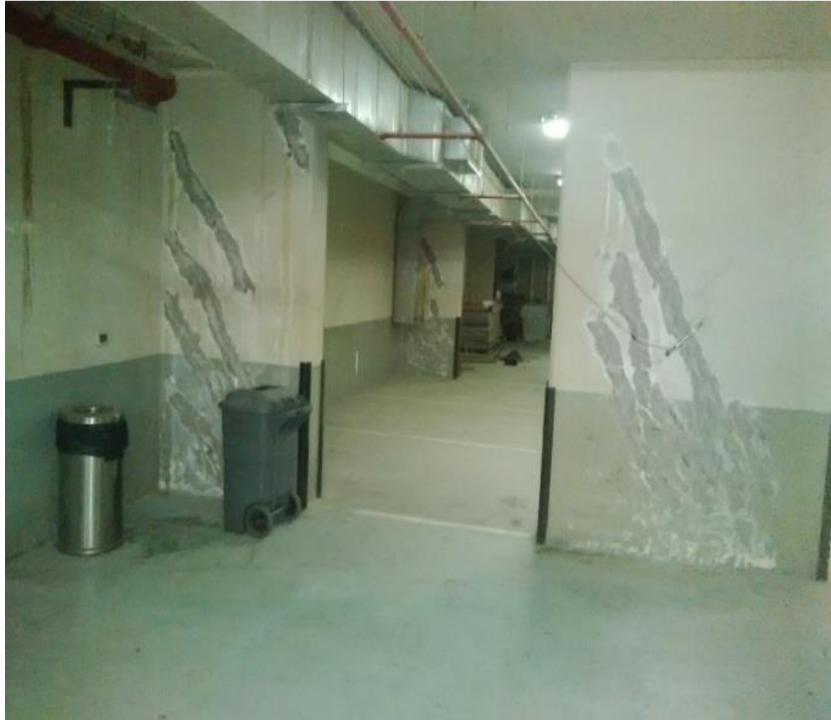
Figure 10: visible cracks and monitoring of cracks
