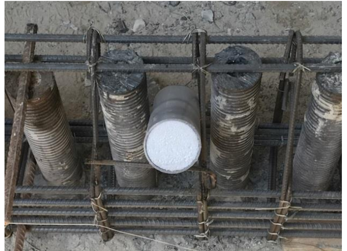
Figure 33: preparation of temporary shoring wall top beam and the sleeve for the anchor to avoid drilling through the reinforcement steel
