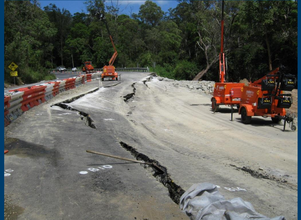
Cunningham Highway Rainfall/floods – ex Tropical Cyclone Yasi – Dec 2010/Jan 2011
