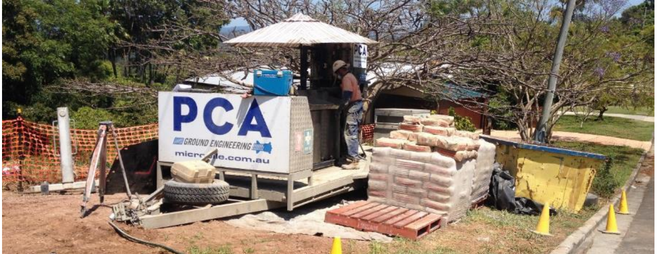
Photograph 4. Grout mixing plant at crest of hill on neighbouring lot to the west
