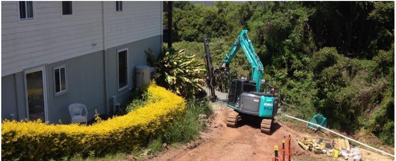
Photograph 5. Access track on neighbouring lot to the west. Piling in progress in Bay 1
