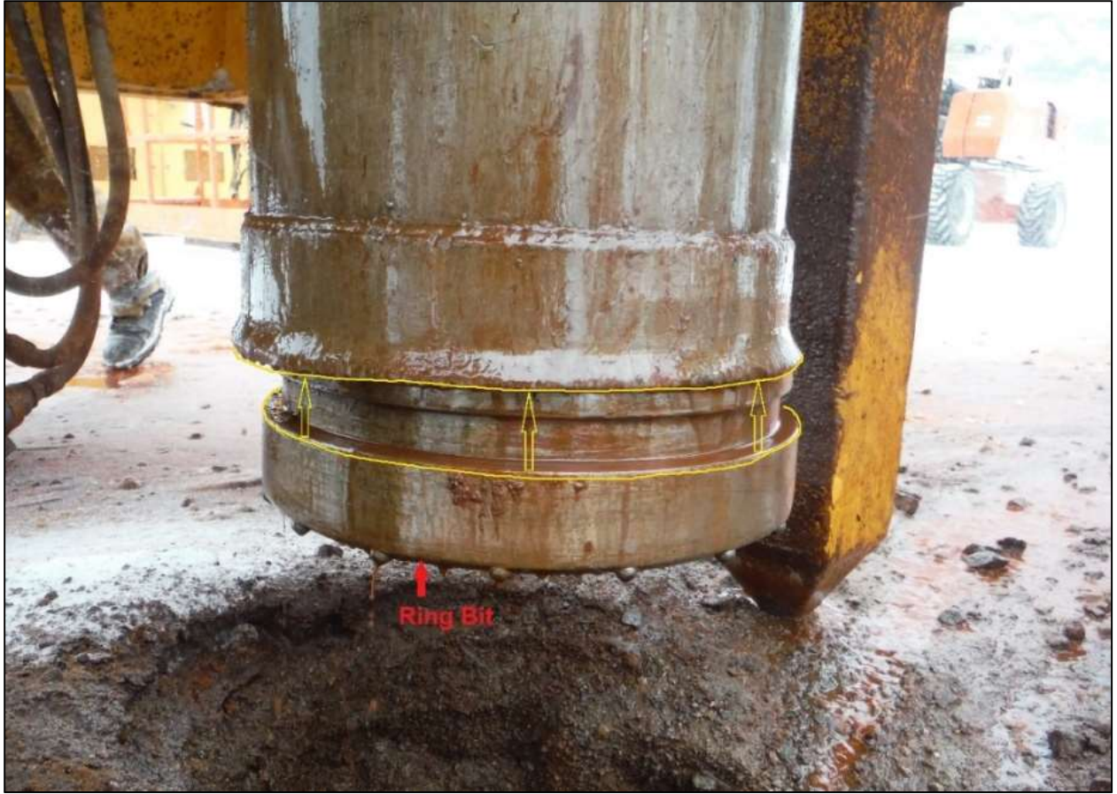
Figure 7: Casing and damaged ring bit after extraction.
