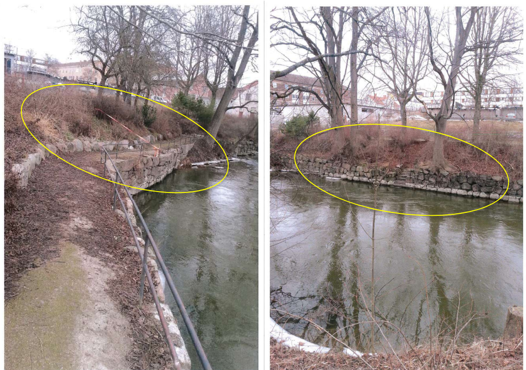
Figure 1 Slope instability signs on the masonry walls (Source: Nyköping City Council)
