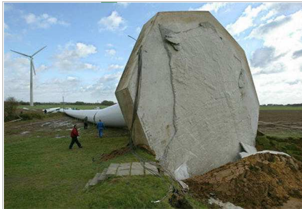
Figure 3. Overturning failure caused by massive rainstorms
