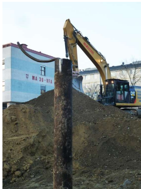
Figure 2 – excavated pile after 30 years of use
