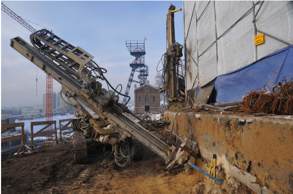
Figure 13. Installation of micropiles anchoring the palisade along MS-15; in the background, building MS-8 and hoisting tower MS-79
