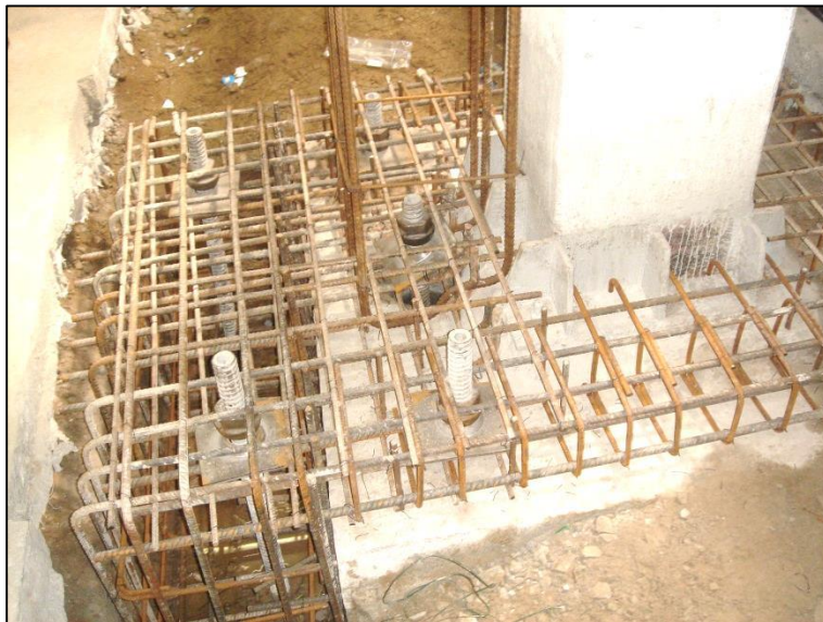
Fig. 5 Scheme with additional supports beyond the block foundation, apparent mounting irons of the additional precast column
