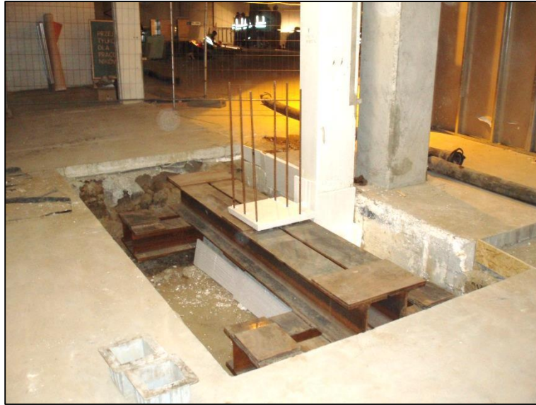
Fig. 6 Transfer of the loads to 4 micropiles (Ti52/26), independent of the existing foundation
