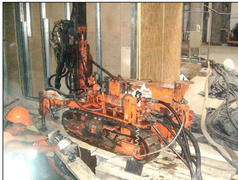
Fig. 9 Injection micropiles inside the building with the use of miniature drilling rig
