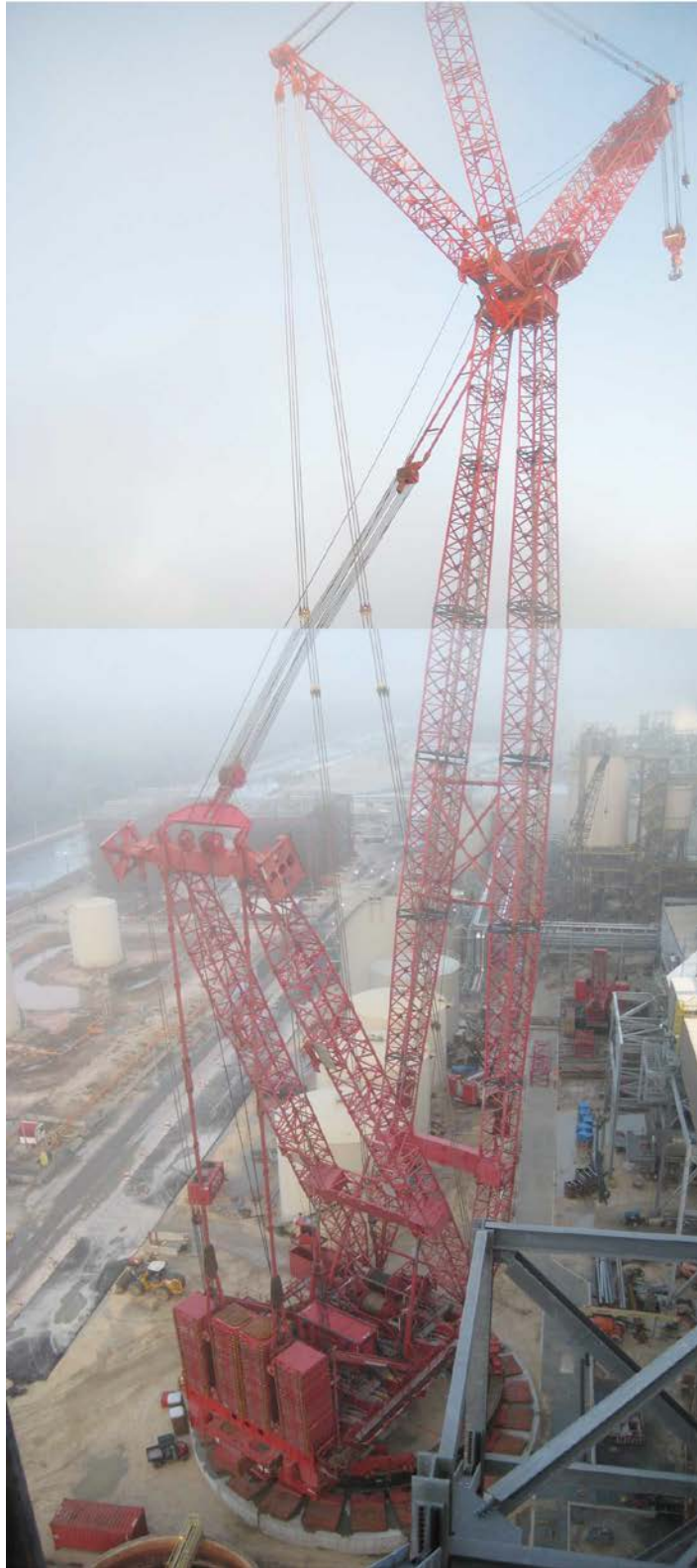
Figure 14. Mammoet PTC ring crane in operation, supported by the value-engineered micropile foundation.
