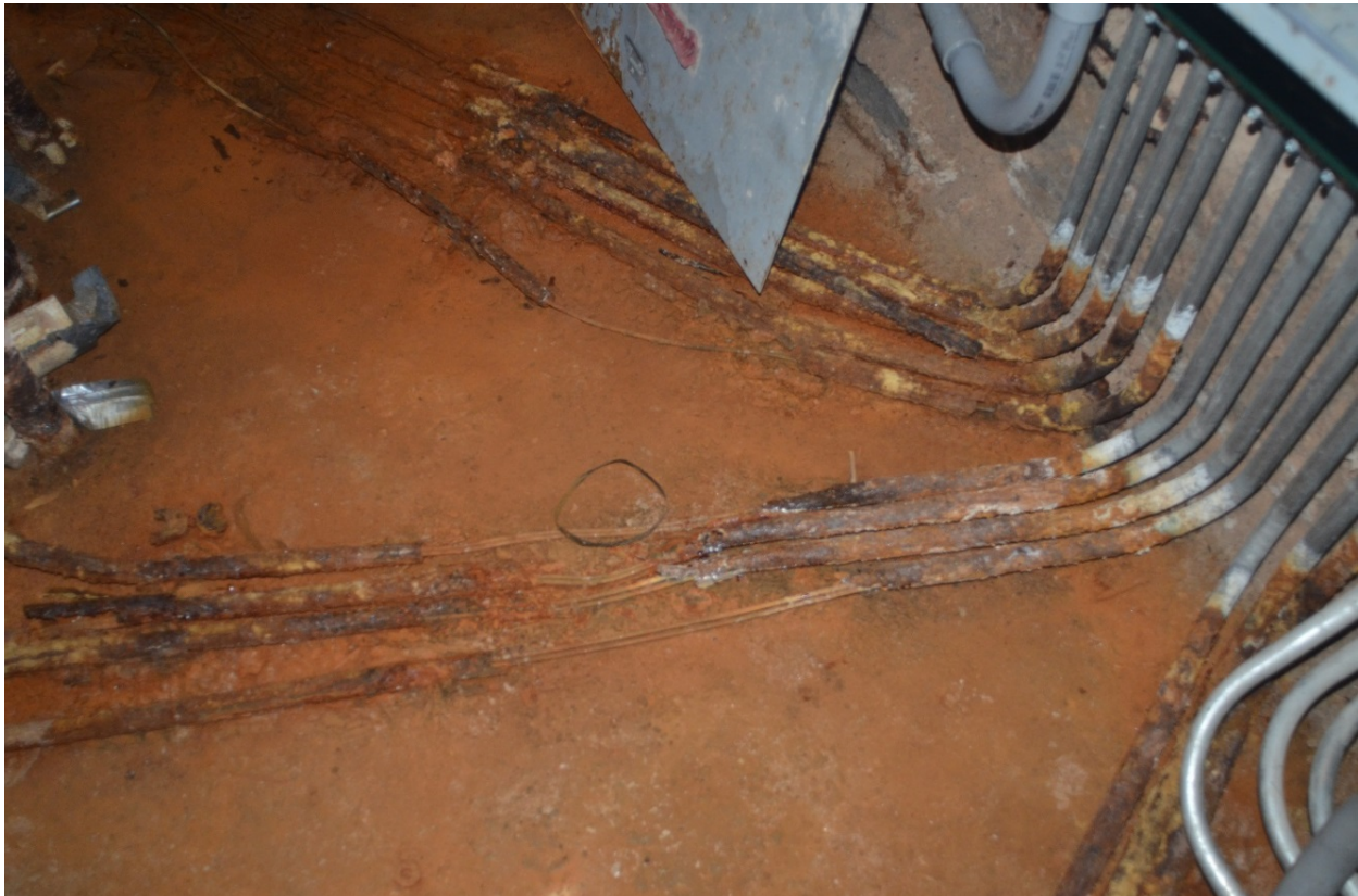
Figure 7 - Steel conduit consumed by corrosion (12/12/2013). Data logger-5 mounted on the south wall of the west elevator.
