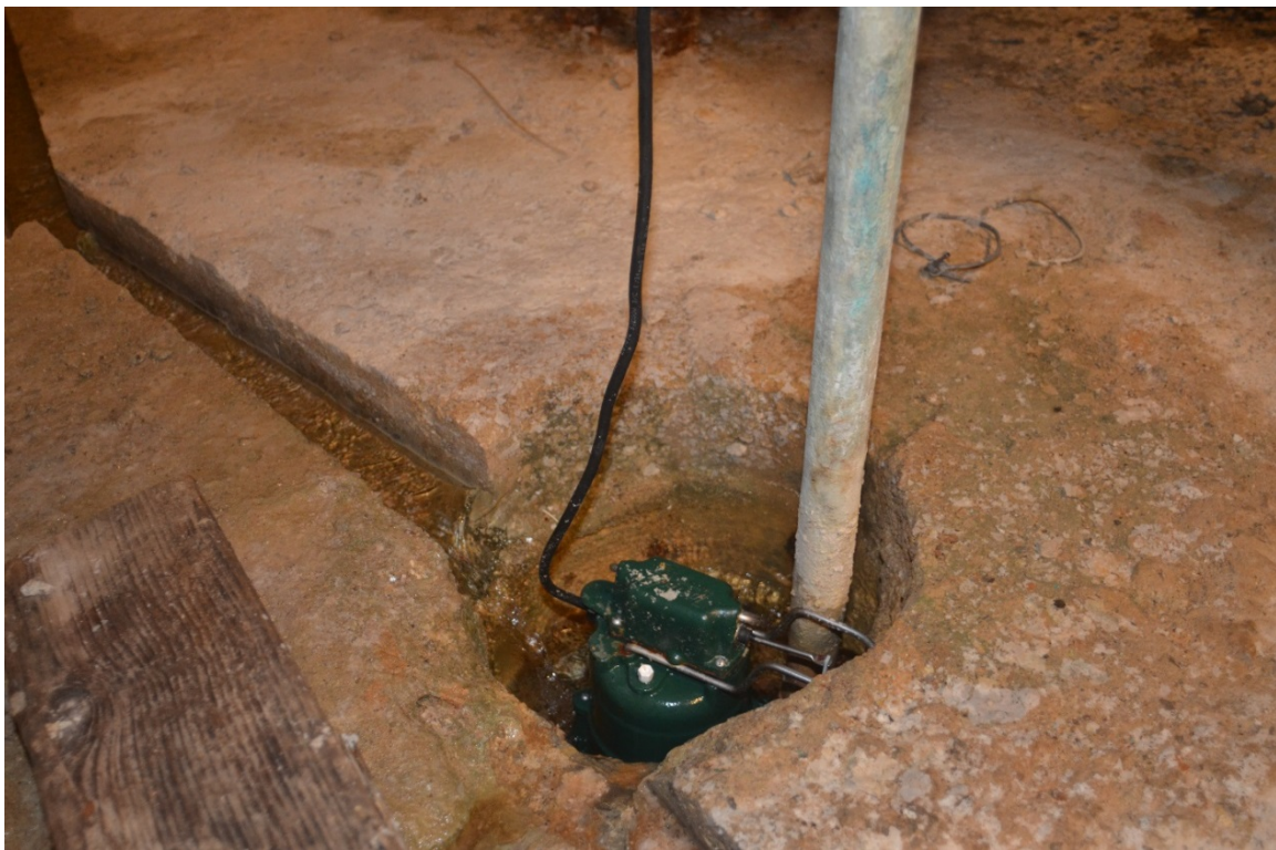
Figure 6 - Sump and pump operating at approximately 1-minute cycle.
