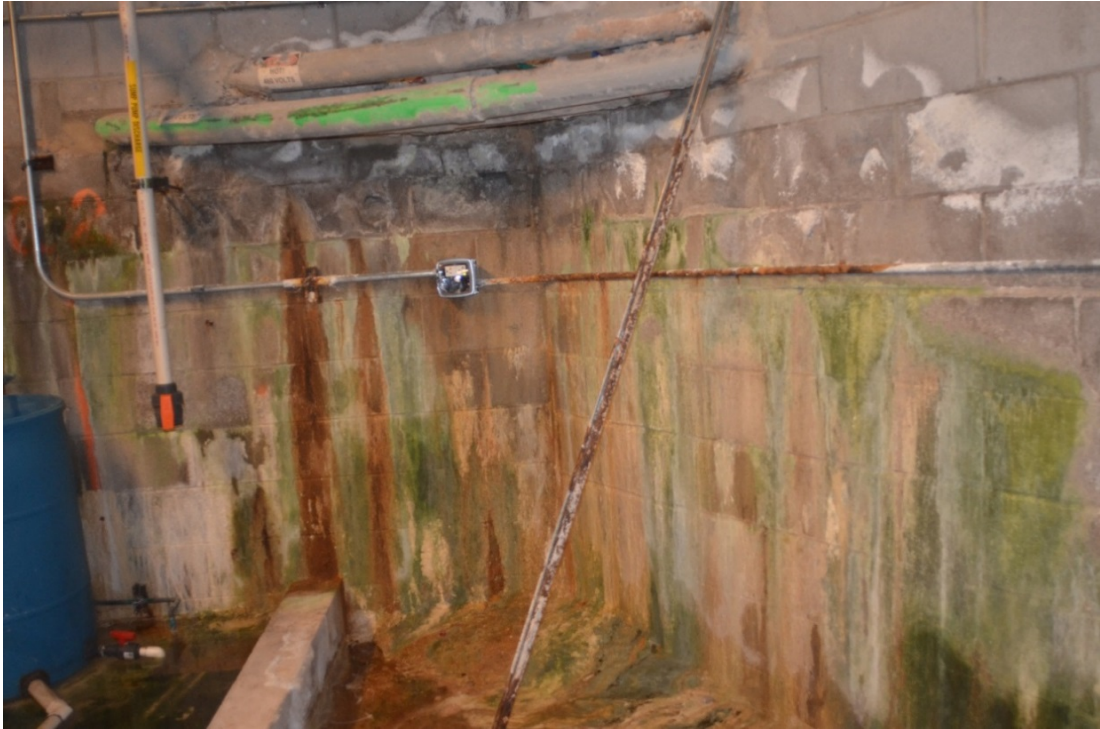
Figure 5 - Seepage and staining, from leaking utility lines.
