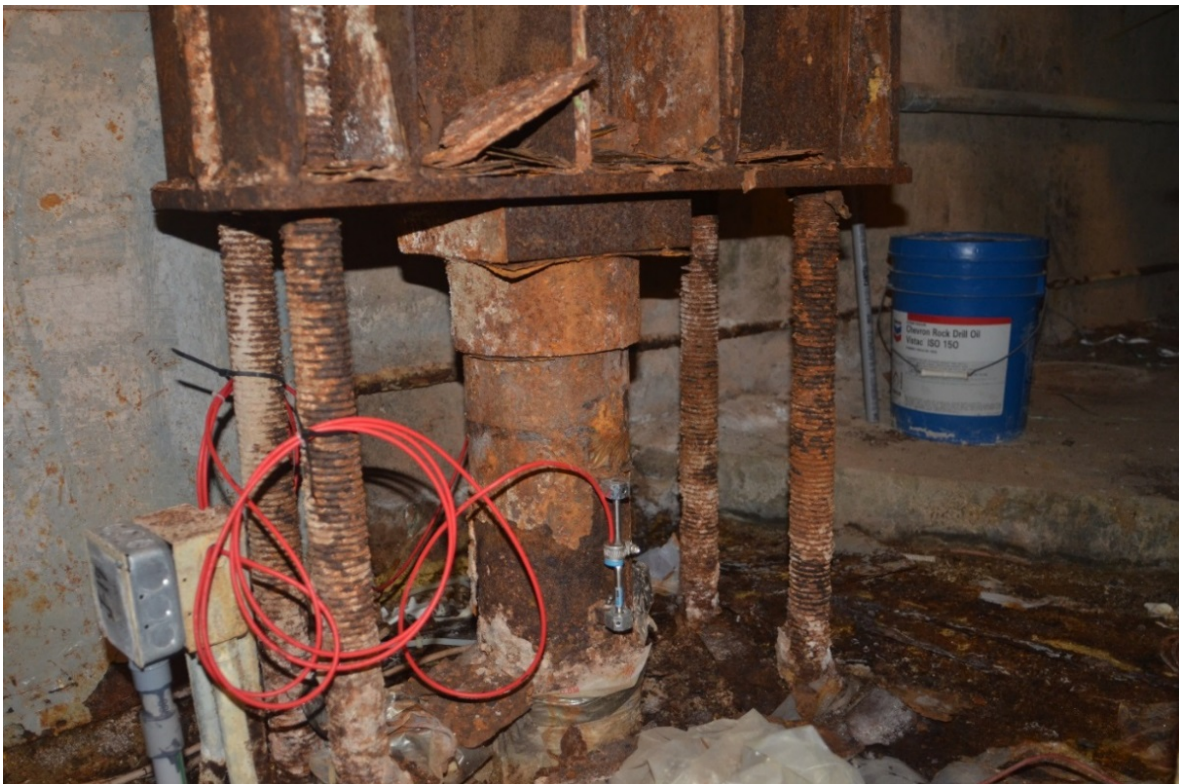
Figure 12 - Micropile J19, 12/12/2013 with replacement VWSG's
