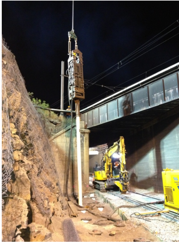
Figure 11: After being lifted into the predrilled hole the hammer is lifted onto the pile for driving.
