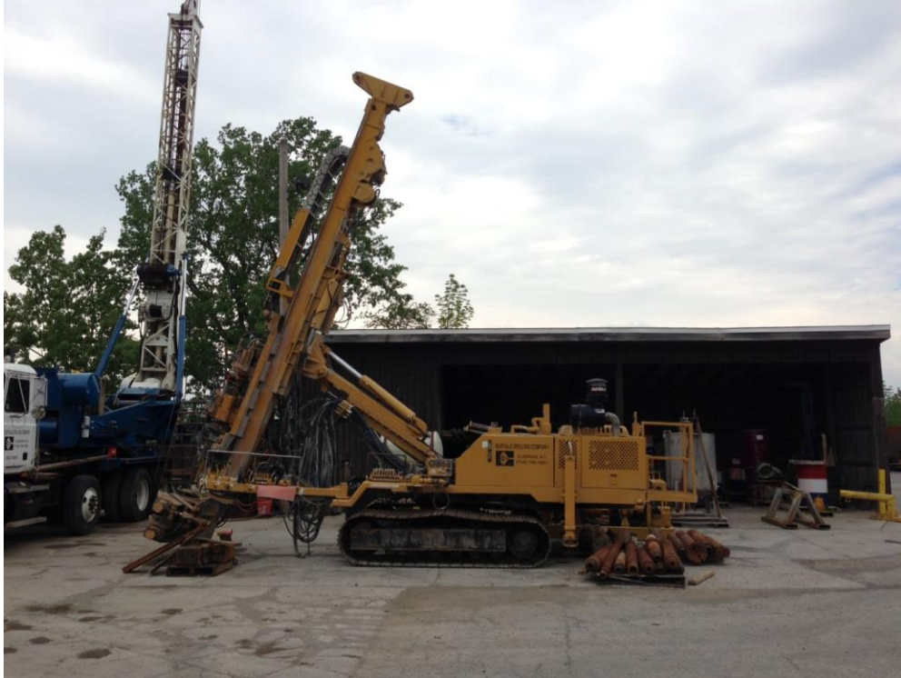
Figure 14. Davey Kent 725 drill rig used for the micropile construction owned by Buffalo Drilling Company, Inc.
