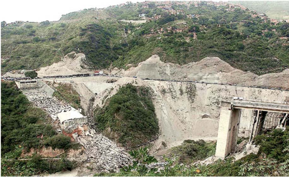
Figure 6. Viaduct after collapse.
