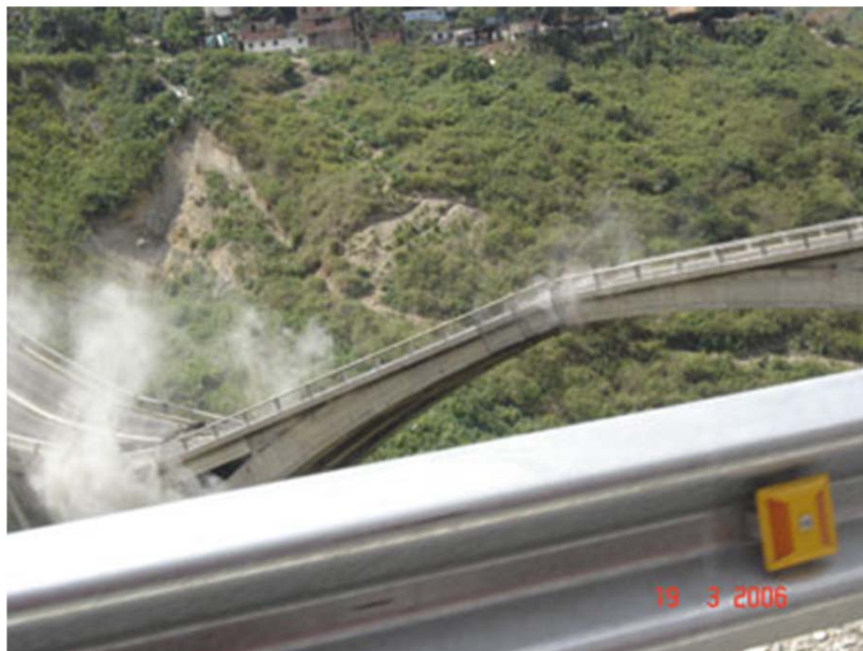
Figure 5. Moment of collapse. Photo by A. Fonseca.
