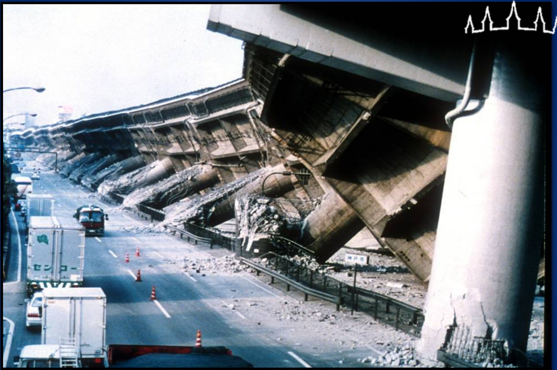
Hanshin Expressway (Hyogo Ken – Nanbu Earthquake 1995)
