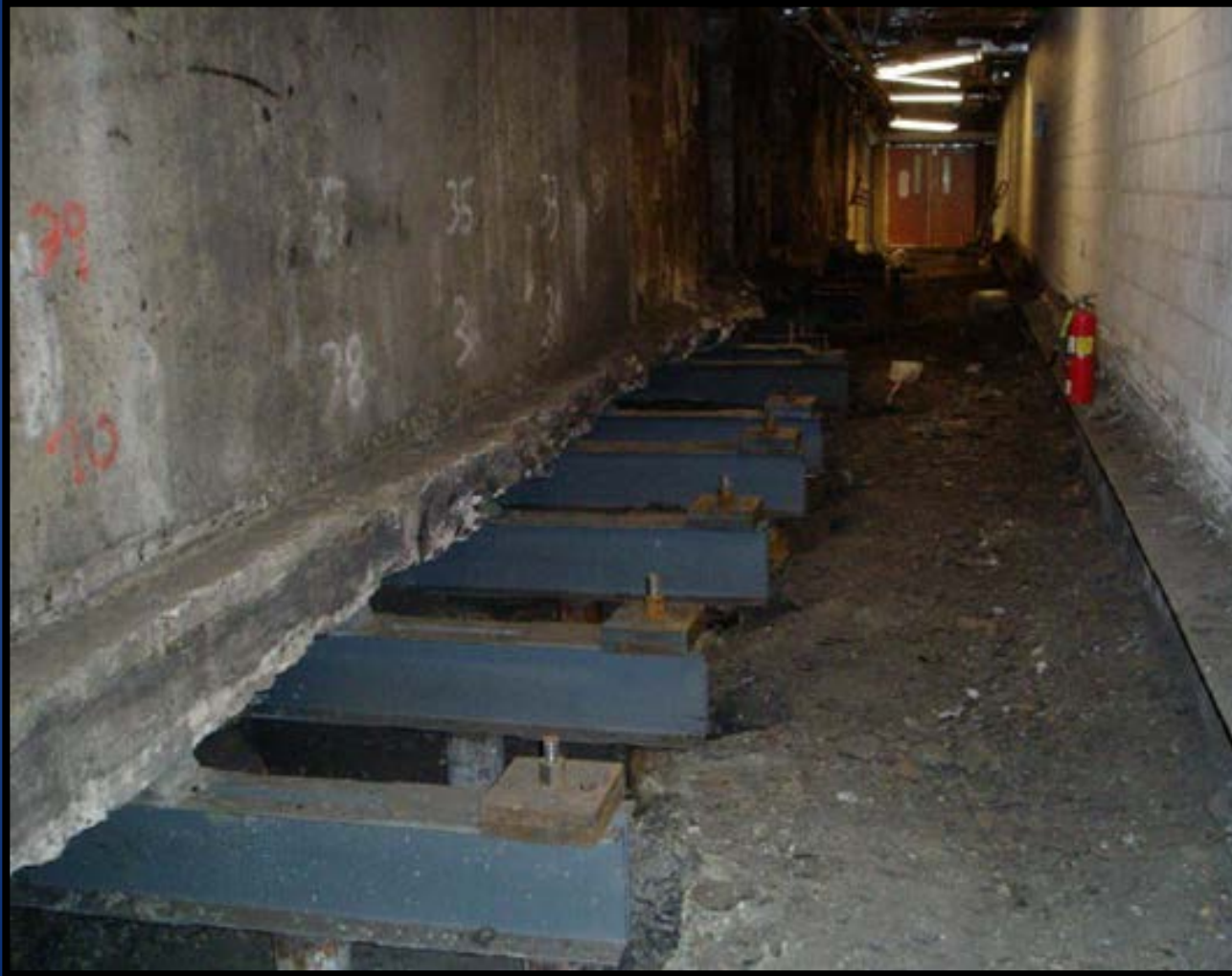
Cracked floor slab, displaced concrete walls and spread footing
