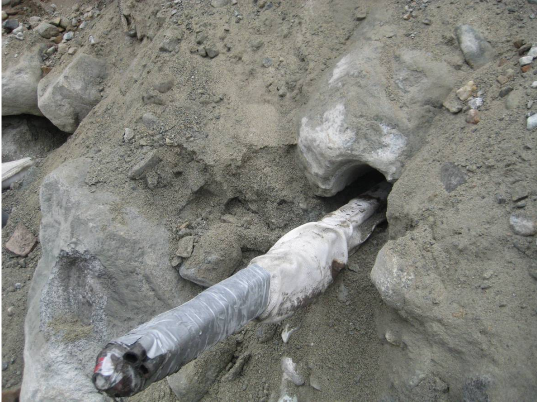
Figure 19. The anchors were installed through the overburden which consisted of very various materials.
