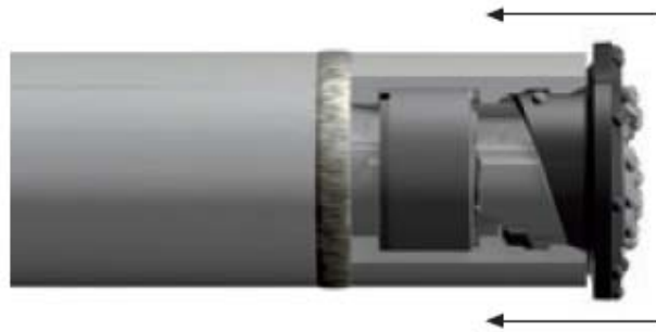
Figure 10. Pulling the drill string backwards to lock the drive ring to the casing extension.
