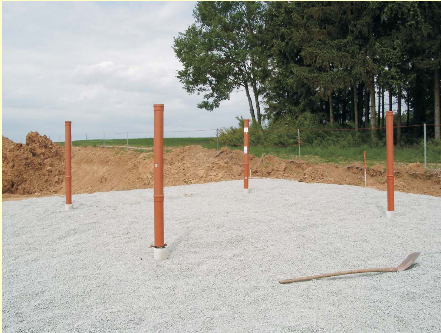
Protruding ends of 4 of the 8 test piles with cable protection tubes and gravel surface
