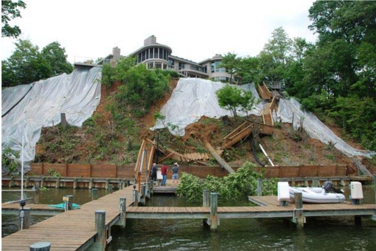
Figure 2. View of the site immediately after the 2008 landslide. Note collapsed staircase and overturned tree (center), collapsed trolley (right), and undermined wooden deck (upper left).
