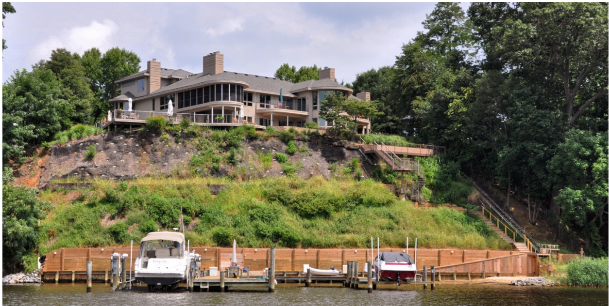
Figure 11. View of the completed stabilization a few months after end of construction. Note slope partially covered in vegetation (Photo courtesy of owner)
