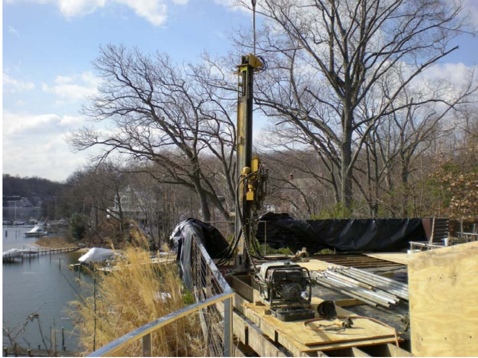
Figure 9. Installation of micropiles through existing deck. The drill mast is suspended from the crane located on a barge below.
