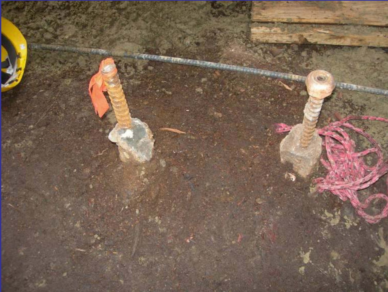
Exposed Piles Notice good grout cover
