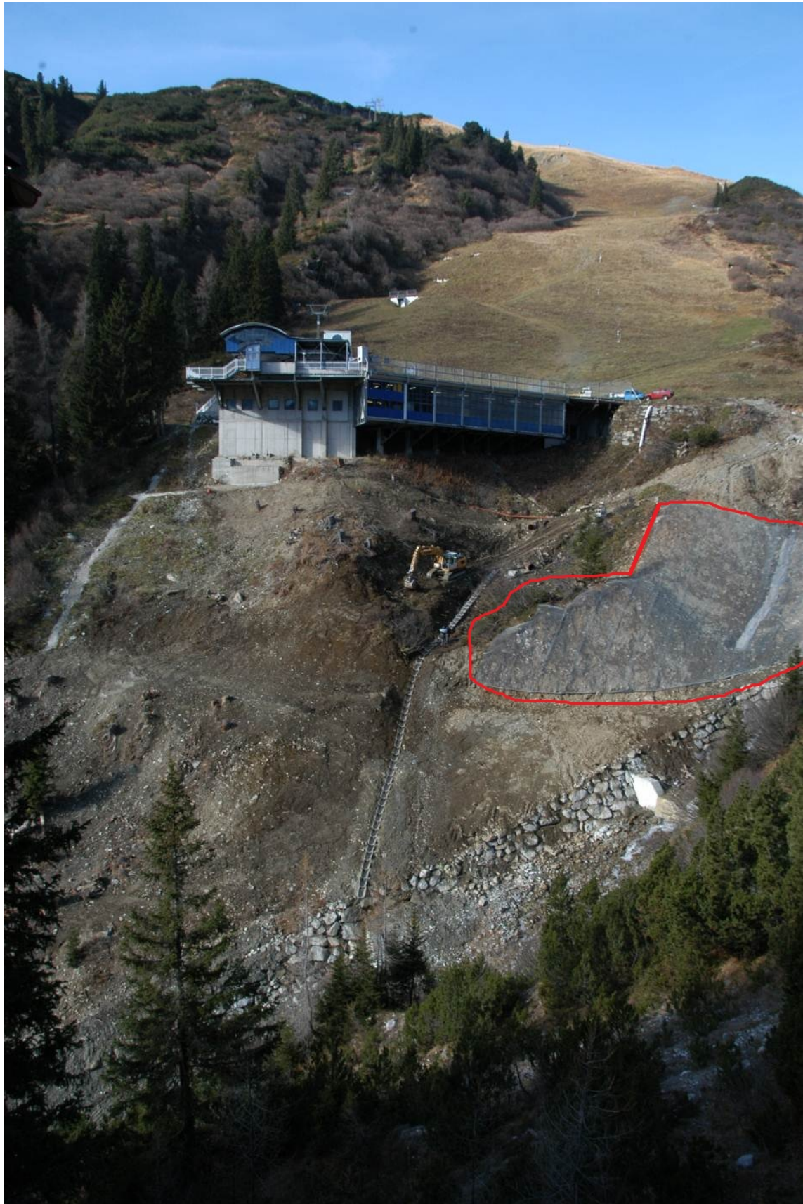
7 finished stabilization work in July 2008 – incl. wire mesh on right hand side
